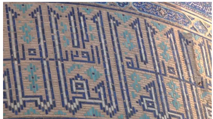
Figure 5. Calligraphic mosaic (cut tile) patterns on the dome tanbur of the Bibikhanum monument.
