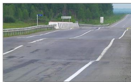
Figure 3. Transverse deformation of the road surface
