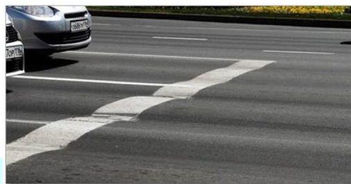
Figure 2. Longitudinal deformations in the upper layer of the road
